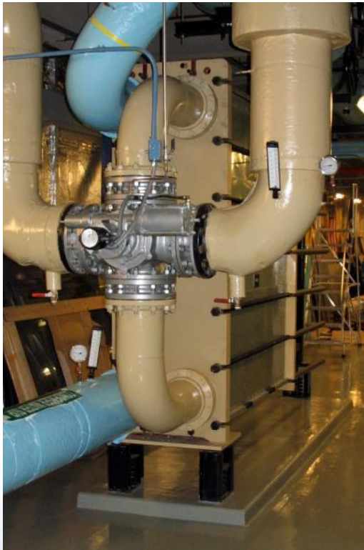
Chilled Water Economizer
