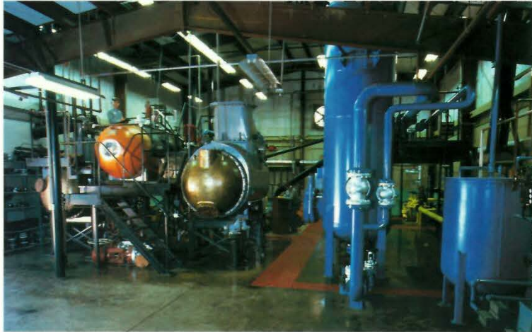
Steam Test Vessel and Condensers
