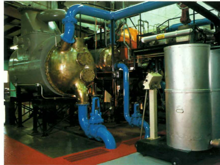
Condensate Collection and Weighing Station
