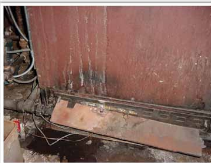
Flame roll-out from boiler jacket, caused by improper venting of flue gasses.
