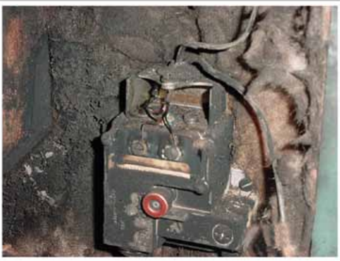
Flame roll-out from boiler damaged the boiler safety control.
