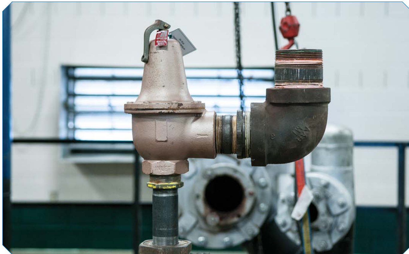
Photo 2 - Section IV hot water boiler safety relief valve
