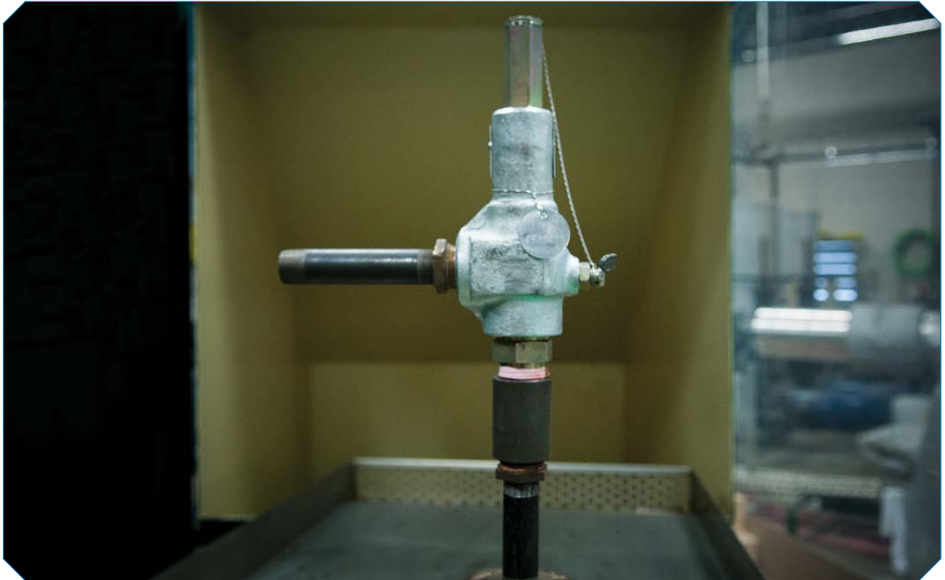
Photo 4 - Section VIII gas service pressure relief valve
