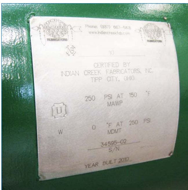
Figure 3: Horizontal pressure vessel nameplate.
