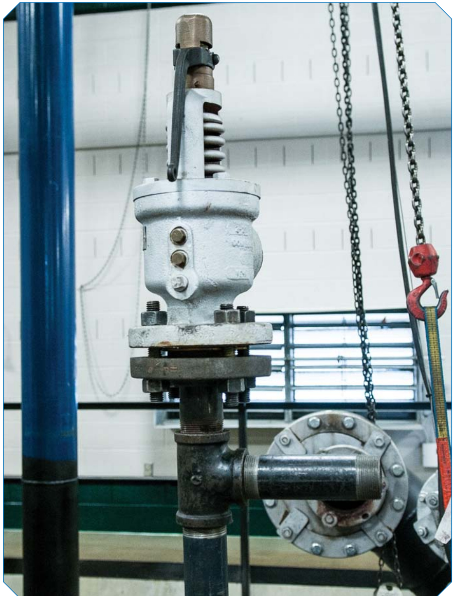
Photo 1 - Section I boiler safety valve
