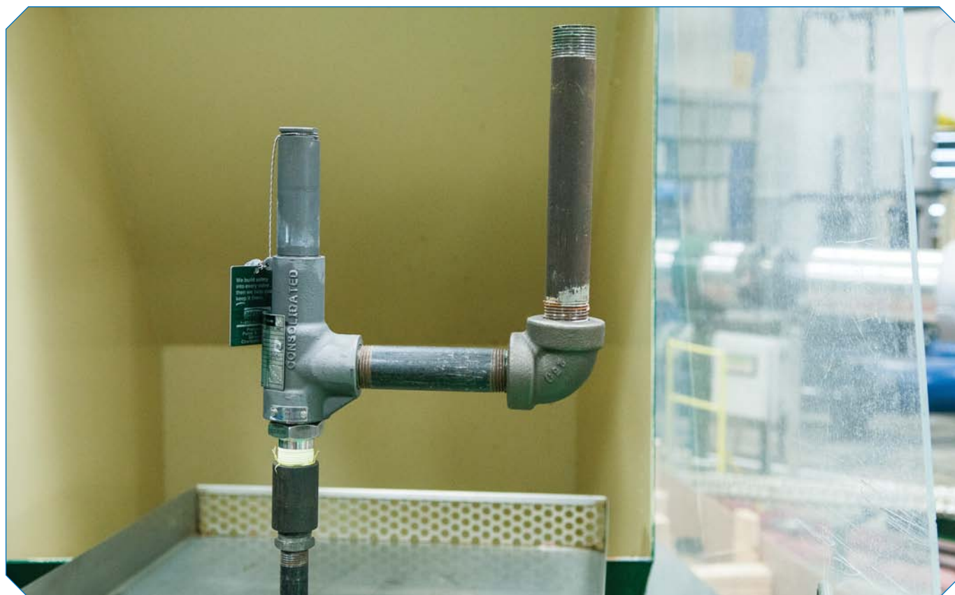
Photo 3 - Section VIII liquid service pressure relief valve
