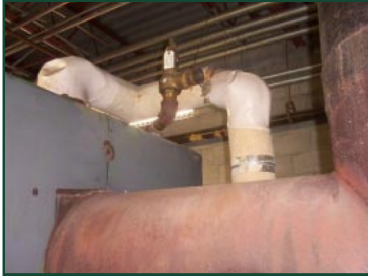
A 30 psi safety relief valve mounted on a 15 psi designed boiler in South Carolina. Discharge side of the safety valve is directed to an unsafe location. ▼
