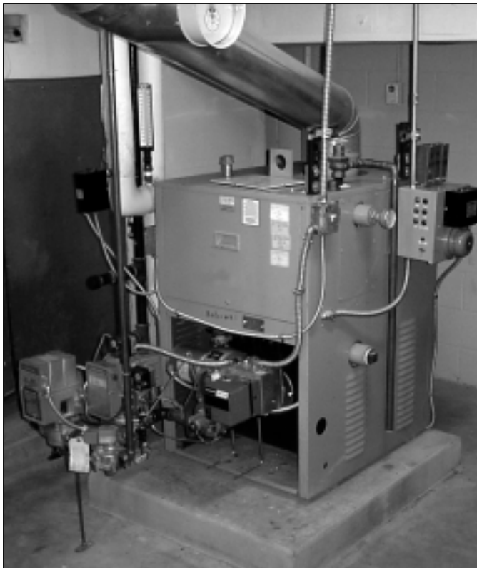
An example of a typical gas burner on a hot water boiler common to malls, schools, and offices.
