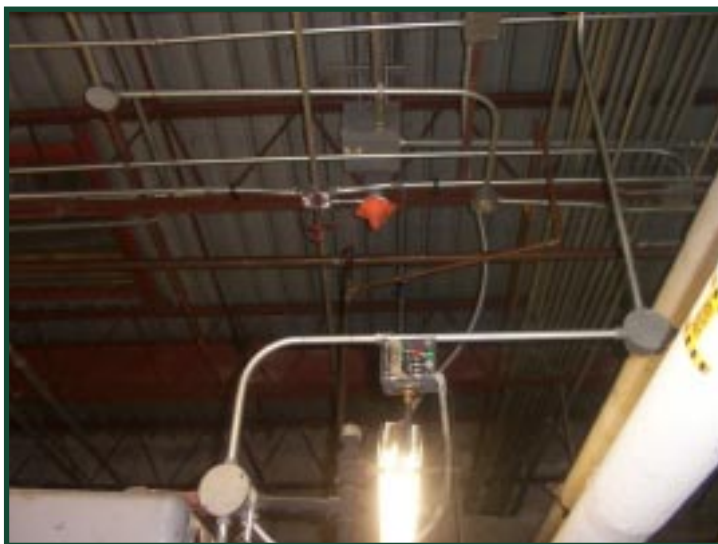
A red plastic device covering the smoke alarm that is above a South Carolina boiler. ▲
