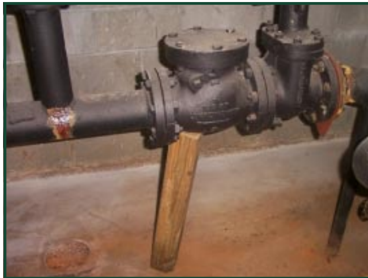
A board supports a pipe connected to a South Carolina boiler. ▼
