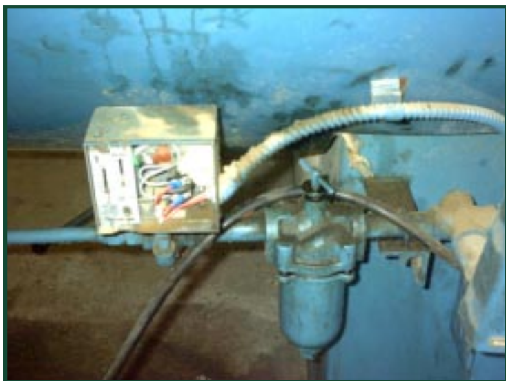
A mercury switch controls the low oil pressure cutoff. This one in South Carolina has been altered with insulating materials preventing the switch from shutting down the boiler in the case of low oil pressure. ▲
