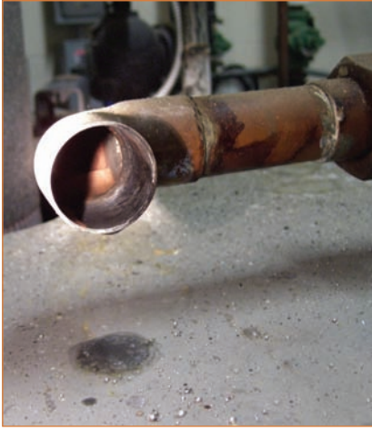
Sweated joints on relief valve outlet.
