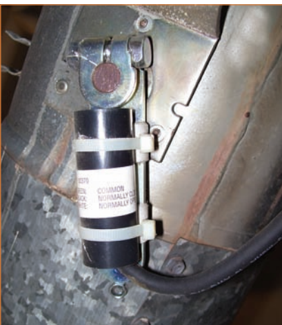
Damper end switch.
