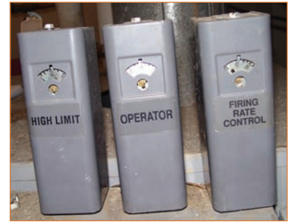
No reset button was found on high limit switch.
