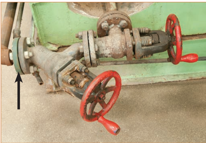
Blowoff valves on 250 psi steam boiler. Code jurisdictional limits include both valves and end at the arrow.
