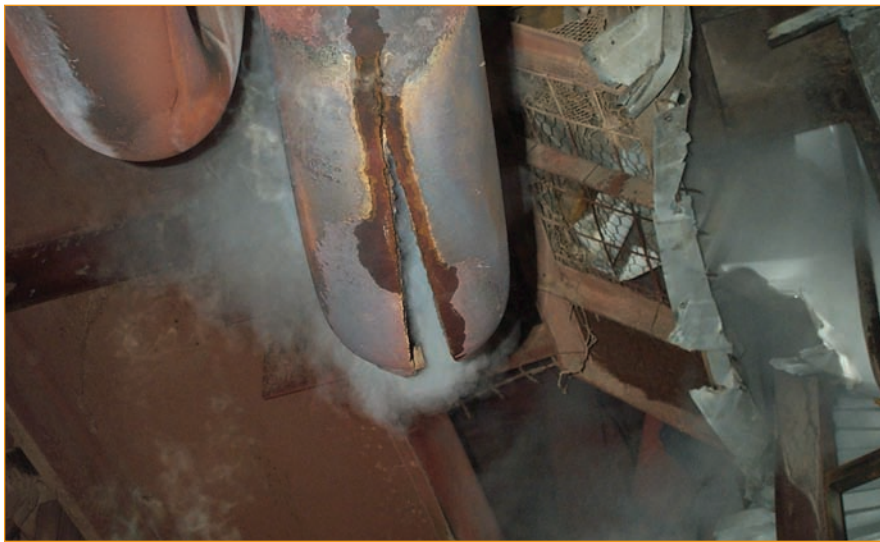
Figure 3: View of one of the link pipe ruptures. Note the axial split, which occurred along the extrados of the bend. Steam is exiting from the rupture after the boiler had depressurized.
