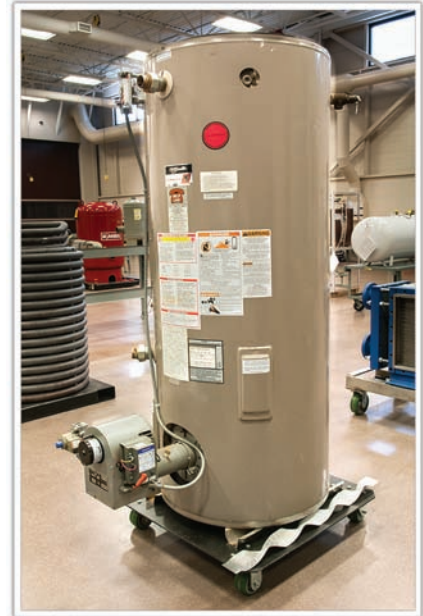
Gas-fired potable water heater, 140,000 Btu/hr firetube construction.
