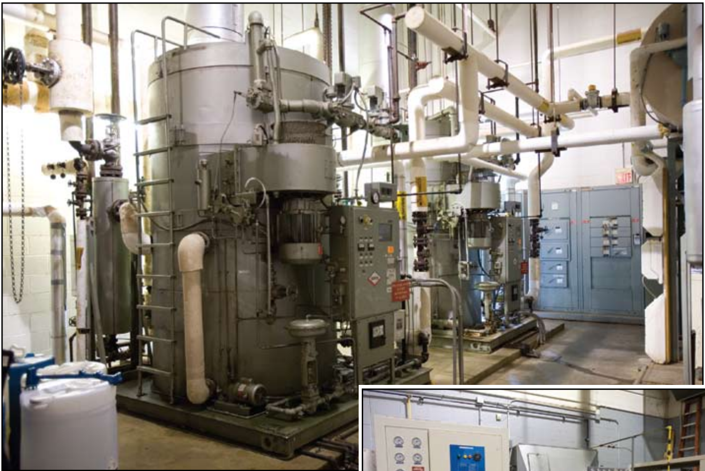
Shown above, two 900 psi steam generators in boiler room behind testing area. High-pressure air compressors (right).
