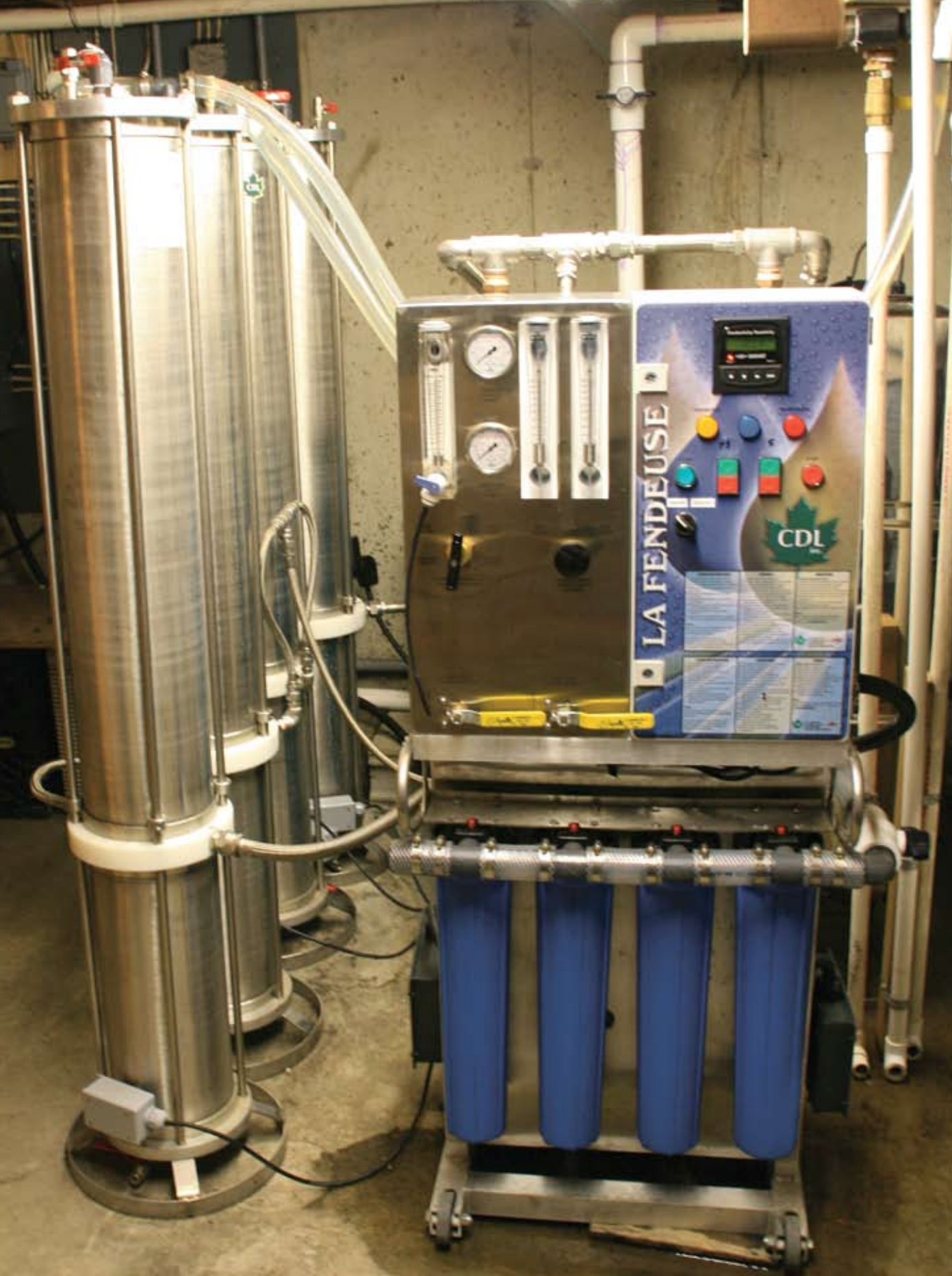
REVERSE OSMOSIS PRESSURE VESSEL
