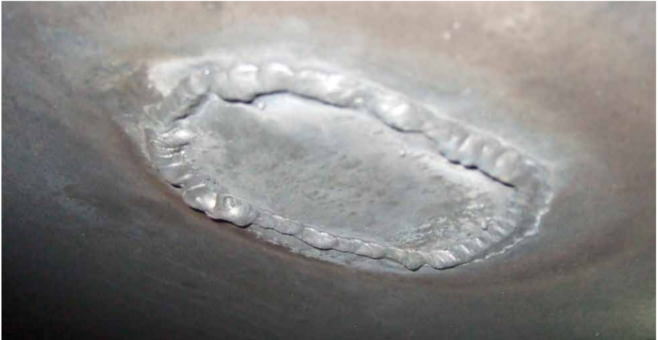
A weld repair by a non-R Stamp facility. Note the poor quality of the weld, including the excess weld material left on the surface. Also note the heat ring around the entire weld – this is from the same person later welding a lap patch on the inside of the cargo tank, because the original weld repair was leaking
