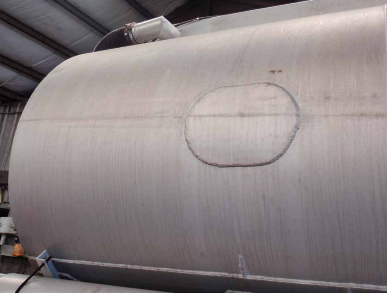
An internal lap weld on a DOT specification cargo tank
