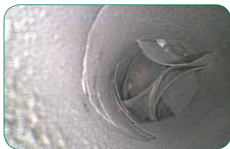
Video probe inside the watertube revealed scale plugging, which led to overheating of the tube.
