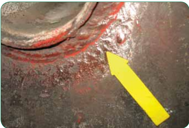
Crack in seal weld of boiler tube to steam drum discovered with MT. This was the result of improper repair procedures.
