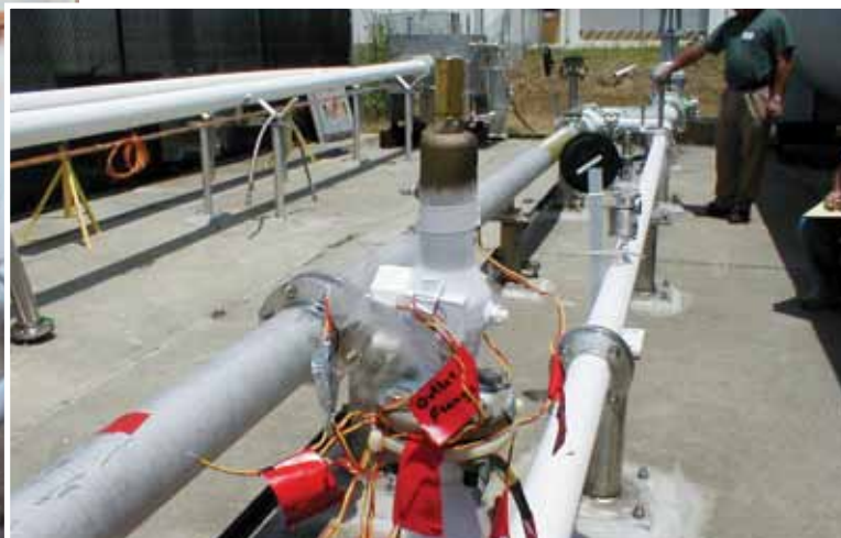
Valve in low-temperature service. (Note lack of frost on bonnet.)
