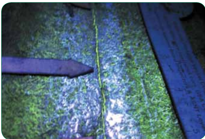
Wet fluorescent MT process showing a crack in a steam drum circumferential weld seam.
