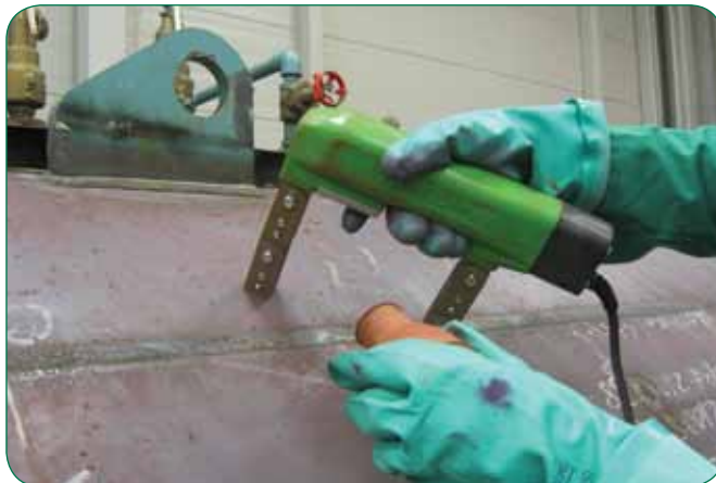
External longitudinal seam of an in-service boiler being checked with magnetic particle examination using an AC yoke with dry powder.
