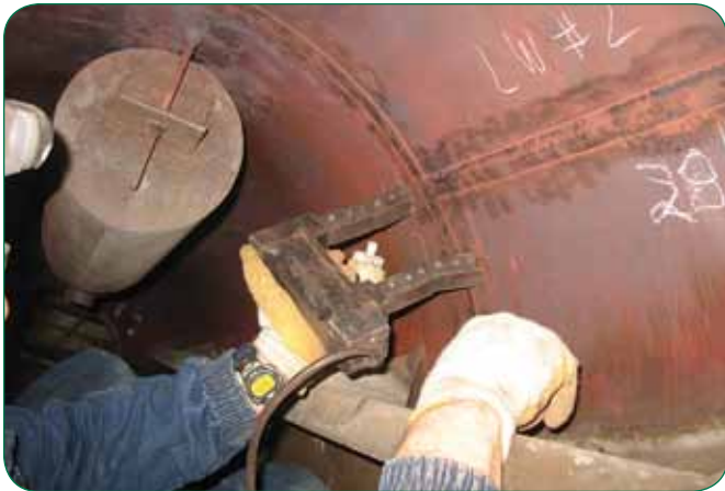
Use of an AC yoke in the MT process to detect fatigue-type discontinuities in welded seams of a steam drum during inservice evaluation.
