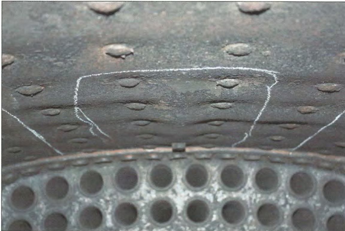
FIGURE OF BULGED STAYED AREA
