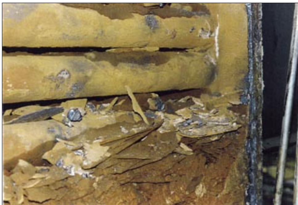
Close-up view showing how scale has flaked off the flue tubes due to overheating. This was caused by the debris-filled water legs considerably reducing the effectiveness of the primary heat transfer surface area (furnace).
